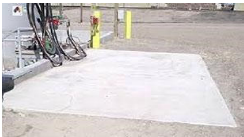
Impervious containment pad
