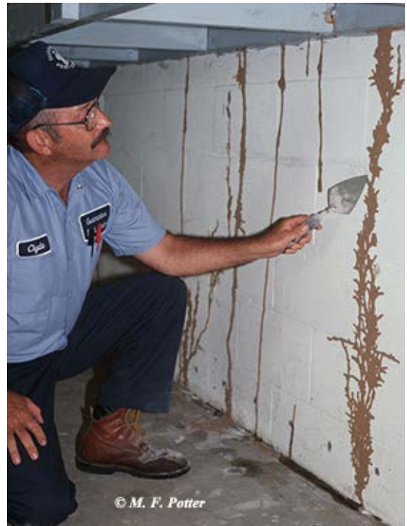
Fig. 4: Mud tunnels are another common indicator of termites.
