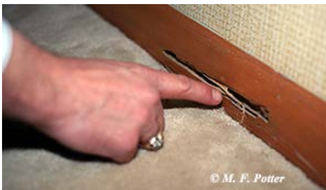
Fig. 7: Termites are cryptic. This damage was discovered when a vacuum head broke through a baseboard.
