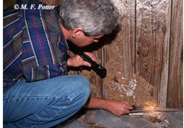
Fig. 1: Termites are capable of inflicting costly damage.
