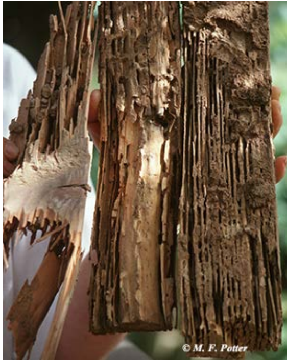
Fig. 6: Termite-damaged wood has soil lining the feeding galleries.
