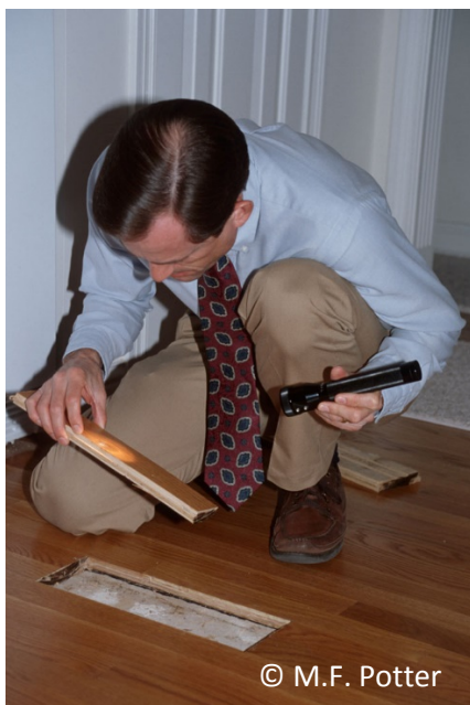
Fig. 7: Replacing small sections of damaged wood can be an effective means of control.
