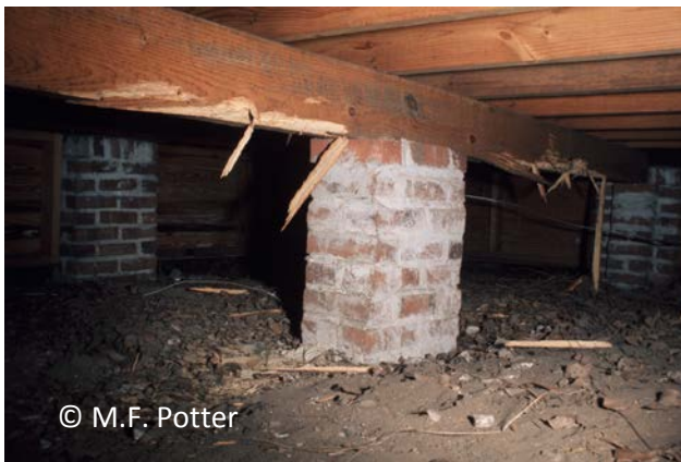
Fig. 4a-b: Anobiid powderpost beetles infest damp areas such as crawl spaces.
